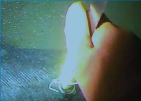
Diver tapping the exposed cable to precisely locate the fault (Courtesy of Energinet)
