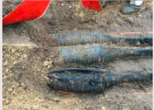
Cable joint with visible damage found at the location of the fault (image 2 - courtesy of Energinet)
